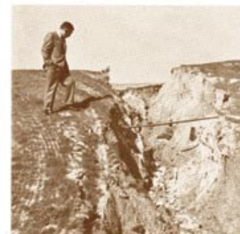
TWO INCHES OF RAIN IN ONE NIGHT ON TOP OF ALREADY SATURATED GROUND CAUSED ENORMOUS DAMAGE. JOE DEEBLE SURVEYS SOME OF THE EROSION. (1969)
